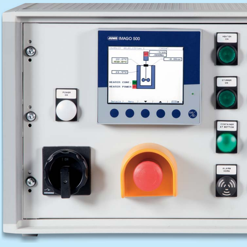
Electrical control box with all options
